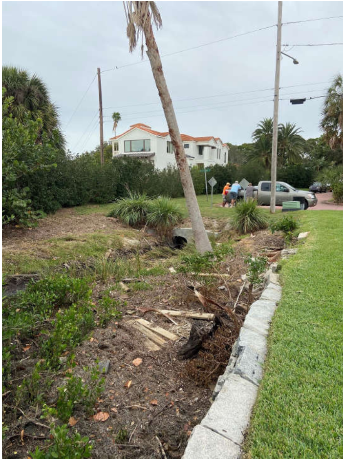
View toward Blossom Way S from encroaching wall along east side of ROW.
